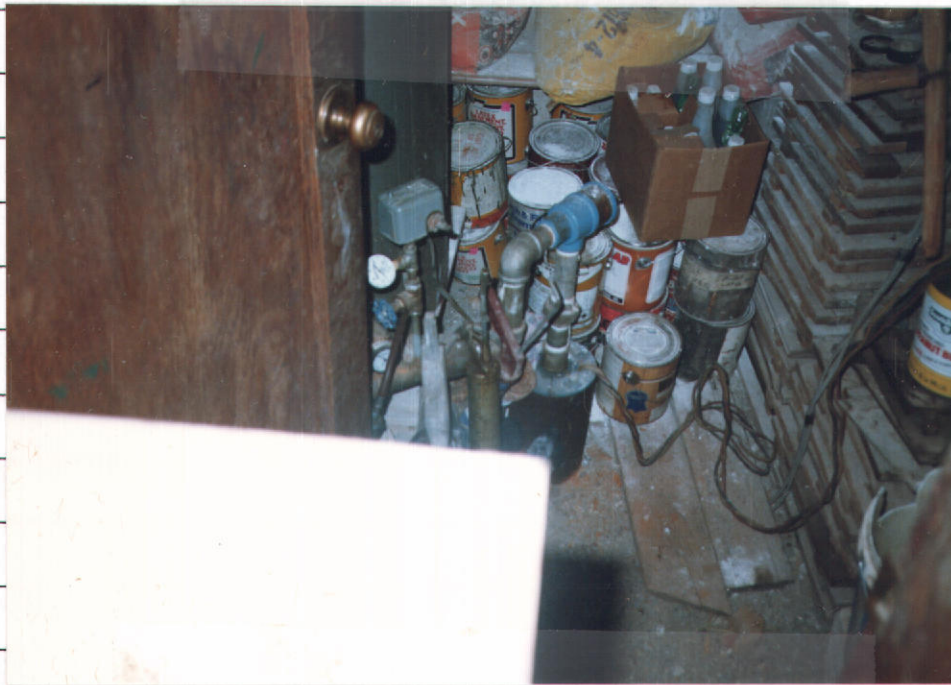
WELL AND WITH BLADDER TANK BEHIND DOOR
