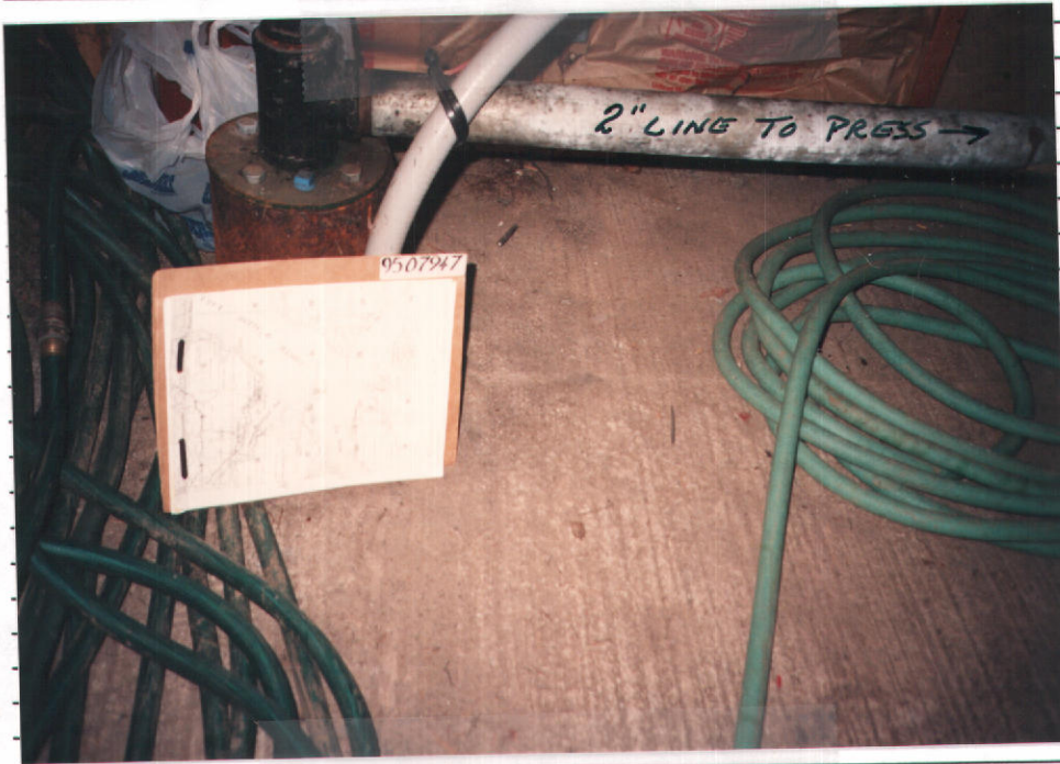
WELLHEAD INSIDE WELL HOUSE
