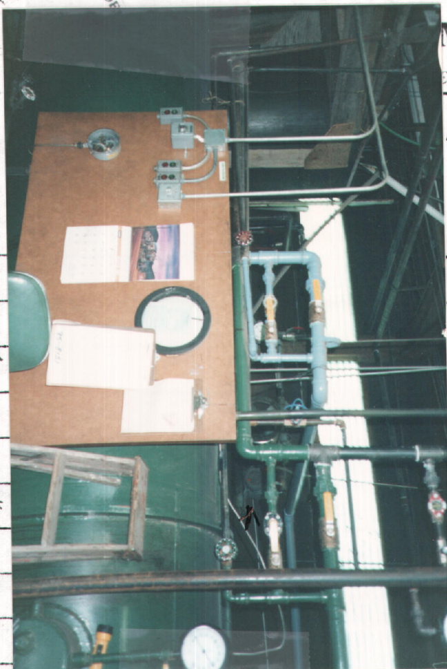
SIDEVIEW 4' RETORTS / MIXING TANK VACUUM PUMP / CONTROL BOARD
