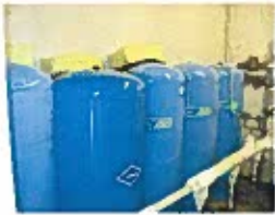
95-8684 Reservoir pumphouse interior.JPG
