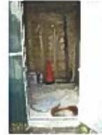
95-8684 Well 2 House view.JPG
