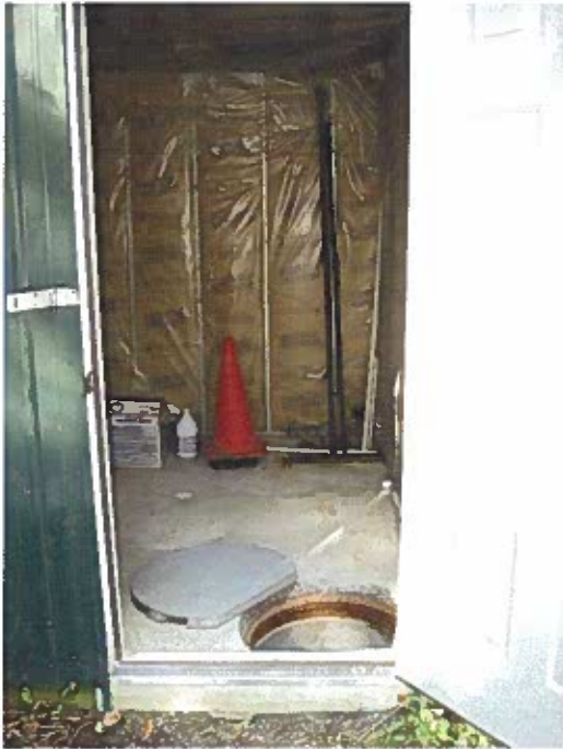
95-8684 Well 2 house view
