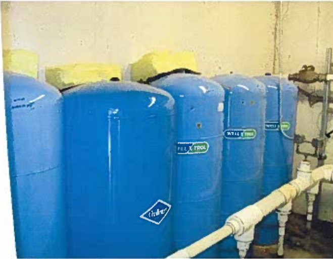
95-8684 Reservoir pump house interior
