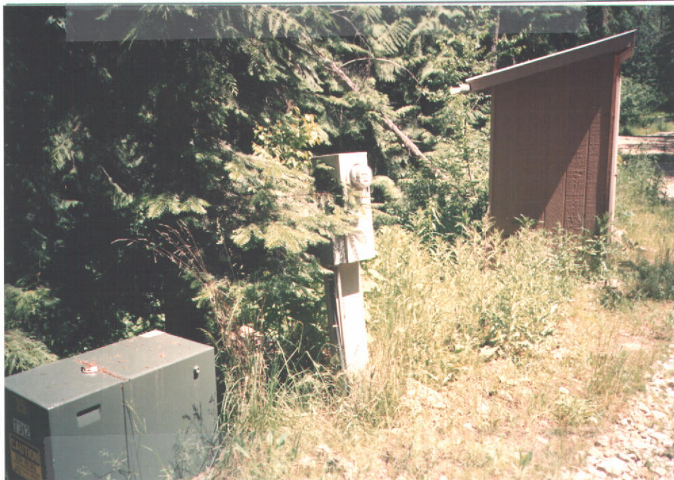
WELL #2 IN WELL HOUSE - LOOKING EASTERLY
