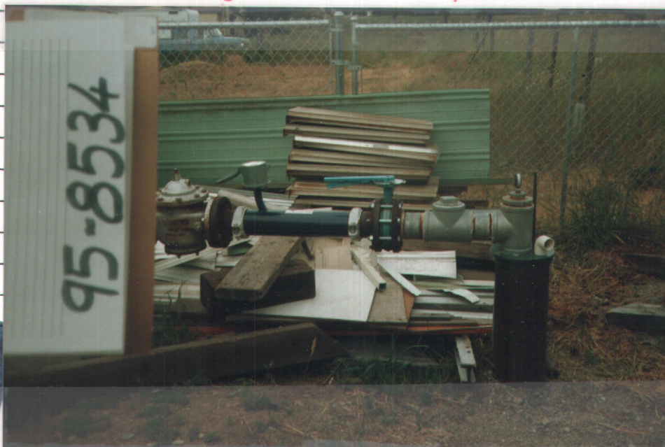
Well and meter
