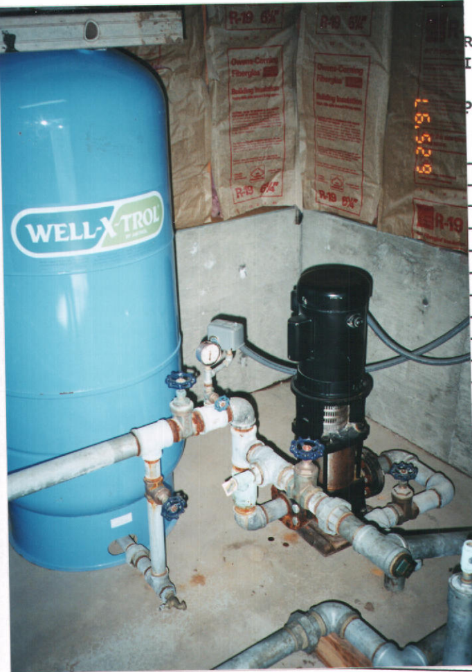
3-HP BOOSTER PUMP
