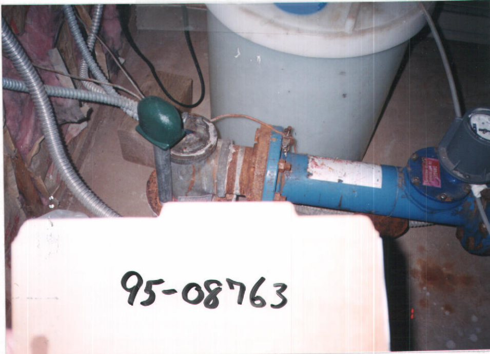
Well # 1 (with meter)
