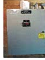
92-7231 Reservoir Telemetry Box.JPG
