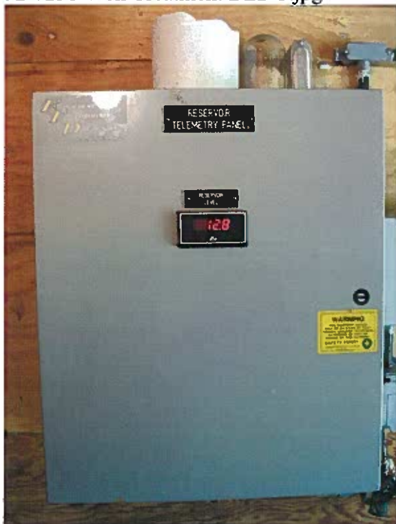
92-7231 Reservoir Telemetry Box.jpg
