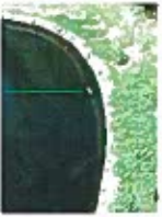
92-7171 Water Exiting Sand Filter Inlet Pipe.JPG
