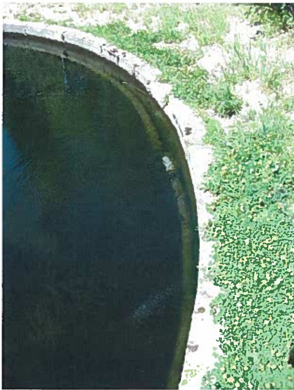
92-7171 Water Exiting Sand Filter Inlet Pipe.jpg
