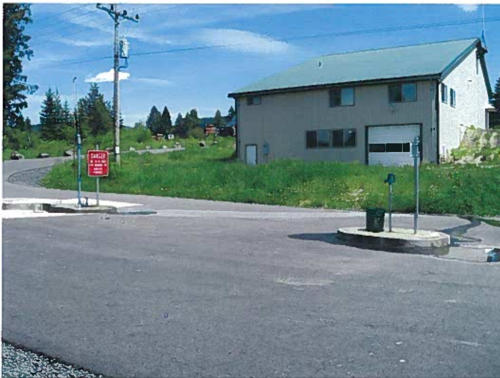
92-7171 Drinking Water & Non-Potable at RV site.jpg
