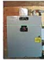
92-7171 Reservoir Fill Control Box at 92-7231 W...
