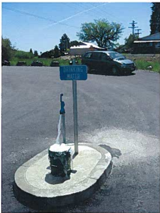
92-7171 Drinking Water at RV site.jpg
