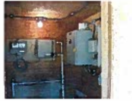
92-7171 Reservoir meter house.JPG
