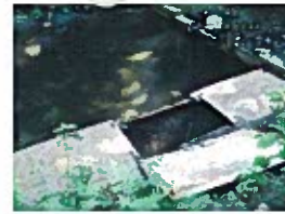
92-7171 Adams CR Pipeline Inlet Top.JPG
