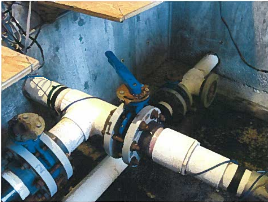
92-7171 Sand Filter to Reservoir Valve.jpg
