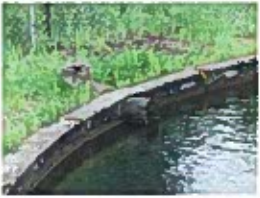
92-7171 Sand Filter Overflow Inlet pipe.jpg
