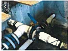
92-7171 Sand Filter to Reservoir valve.JPG
