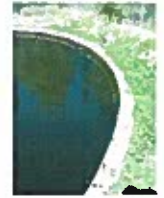
92-7171 Water Exiting Sand Filter Curved Inlet Pipe.JPG
