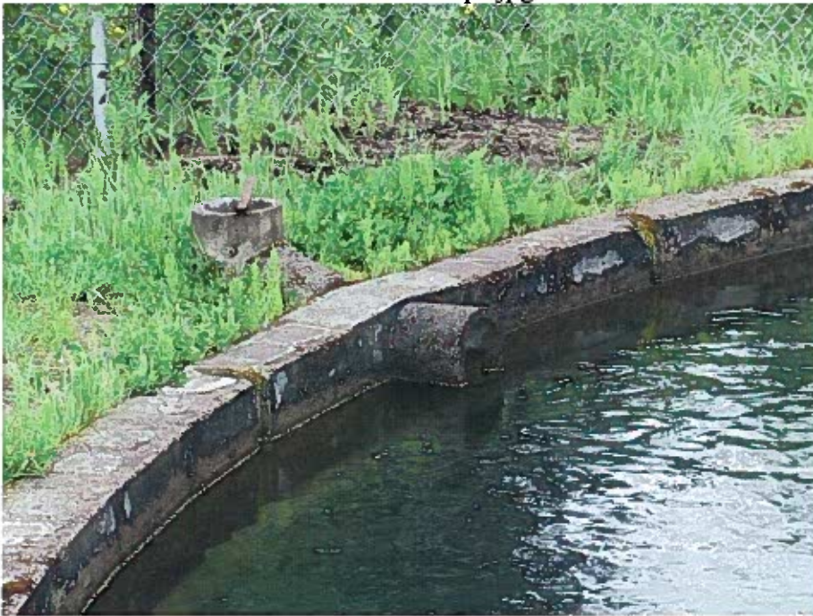
92-7171 Sand Filter Center Overflow Inlet Pipe.jpg
