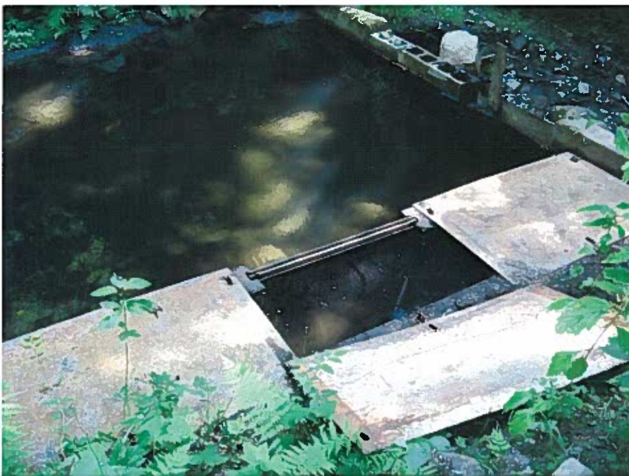
92-7171 Adams CR Pipeline Inlet Top.jpg
