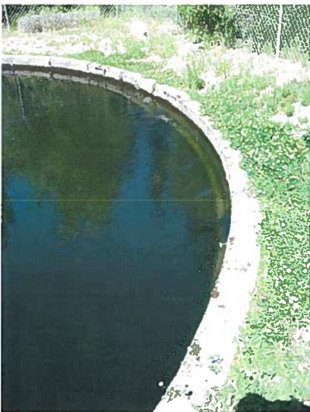
92-7171 Water Exiting Sand Filter Curved Inlet Pipe.jpg
