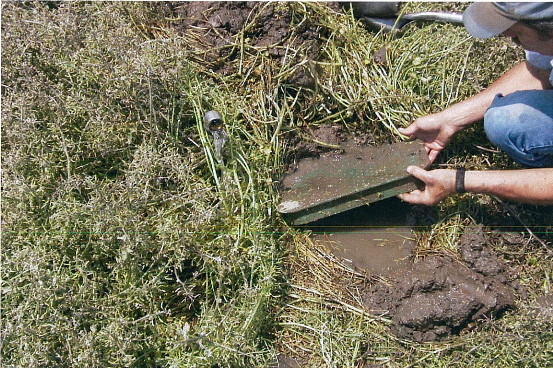
Photo of spring box with a valve inside to control the flow
