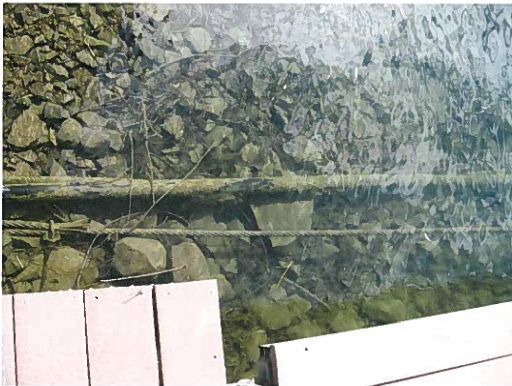
95-9352 Two Inch Water line to Submersible Pump
