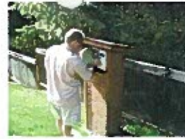
95-9352 Irrigation Electronic Control Station.JPG
