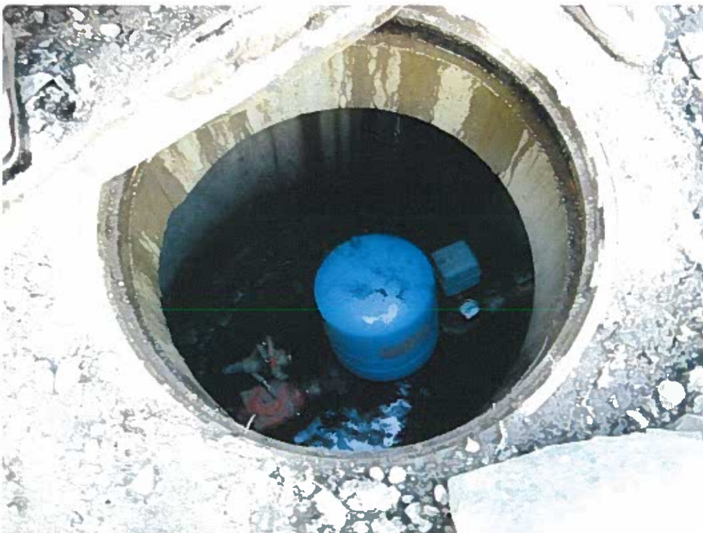
95-9352 Underground Vault with Pressure Tank
