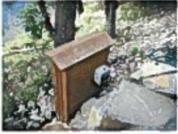
95-9352 Electrical Box at Bottom of Pipeline to Cont...
