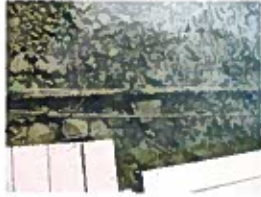
95-9352 Two Inch Water Line to Submersible Pu...
