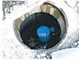
95-9352 Underground Vault with Pressure tank.JPG
