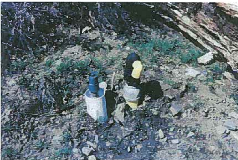
Kenney Crk PL Airvents (left, BLM stockwater PL right, private irrigation PL)
