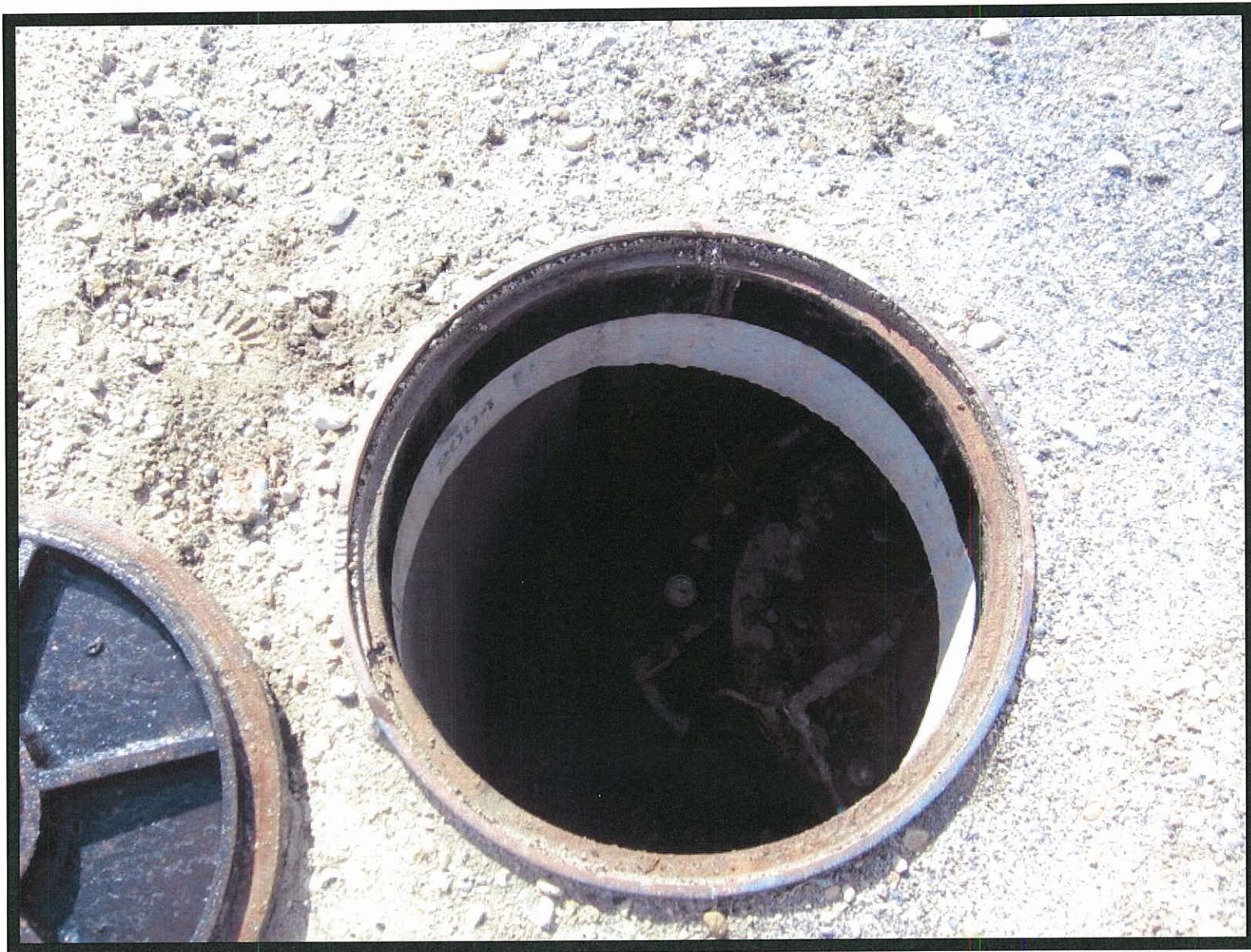
Potable System Connection on NW corner of Iowa Ave and Middleton Rd (other manhole connection is about \frac{1}{4} mile north of Greenhurst Rd located in the center of Middleton Rd)
