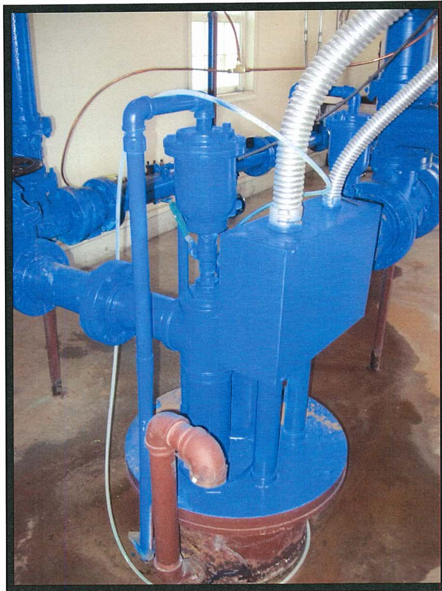
18-inch Well with 30 hp and 100 hp Submersible Pumps
