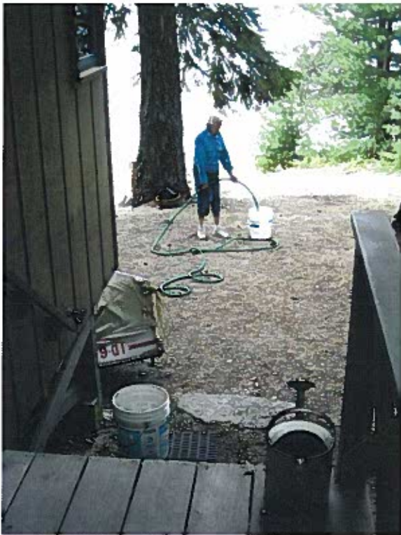
97-7471 Water Flow test at POU
