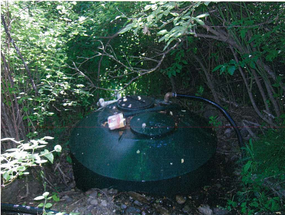
600 gallon domestic water storage tank. Currently water is manually carried from tank to house. Water user hopes to have a pump in place soon to lift water to house.
