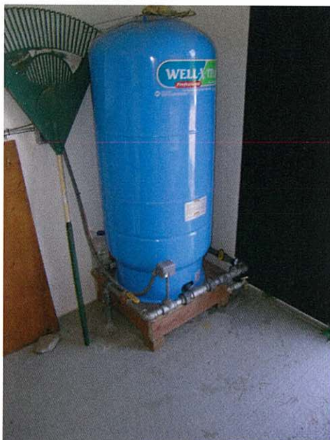
Well pressure tank in Utility Shed.
