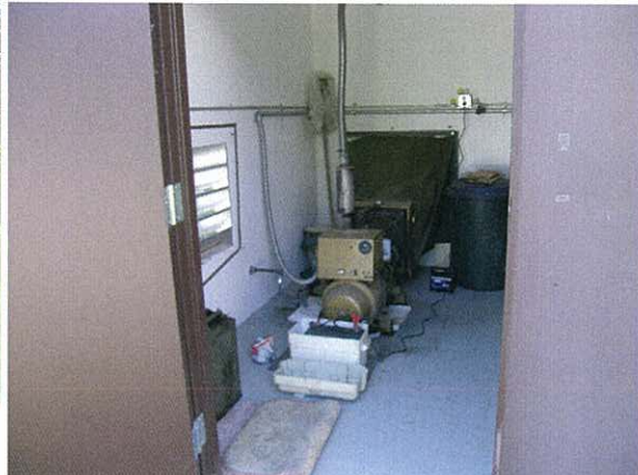
Generator and batteries in Utility Shed.
