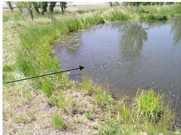
Inlet Discharge into Pond, Fully Submerged.
