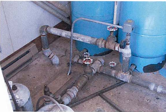
Pic 5. Inside well house 2 west side.
