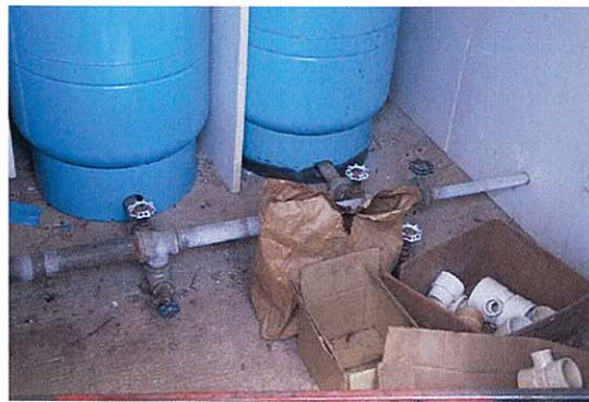
Pic 6. Inside well house 2 east side.
