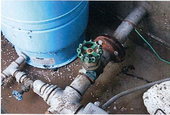
Pic 1. Outlet to system, well house 1
