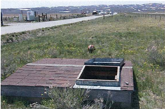
Pic 3. Well house 1 and well head 1.
