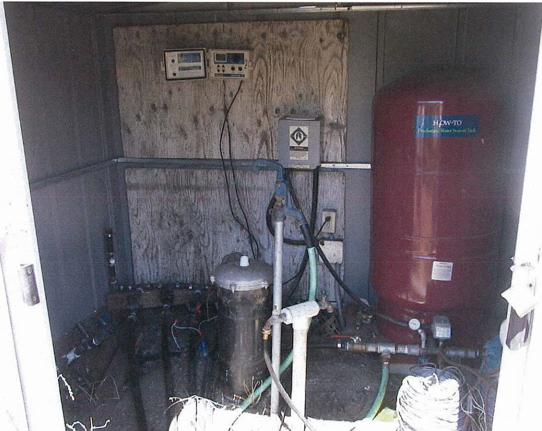
FIGURE 2: Well, pressure tank, control panel, spigots.
