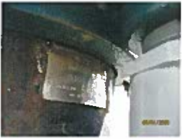
WELL TAG FOR WELL #3 #D0041109.JPG
