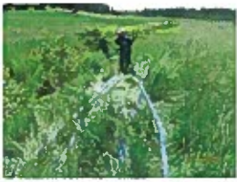
FLOOD IRRIGATION LINES.JPG
