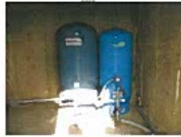
BWS Well House Pressure Tanks.JPG
