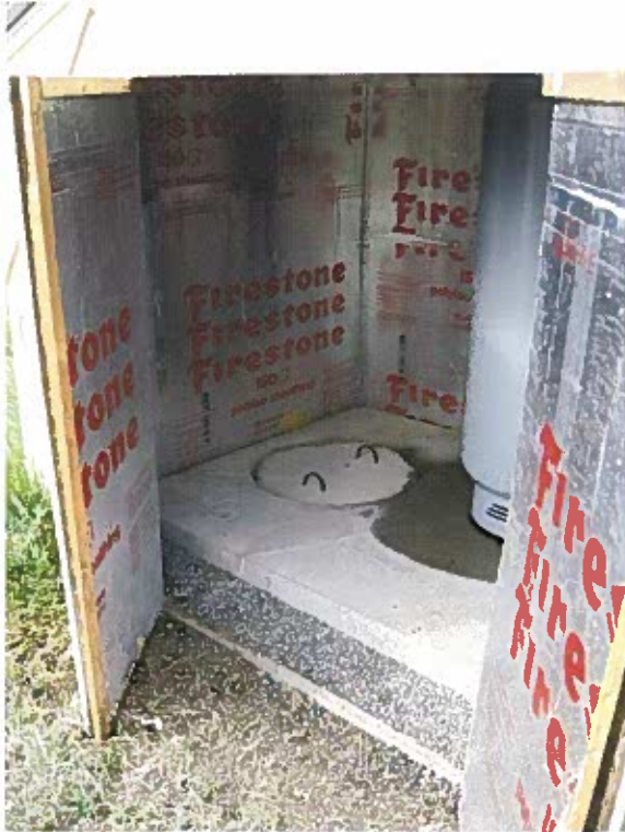
BWS- Non-System Reservoir BLDG Interior
