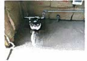
BWS Recordall Flowmeter Location.JPG
