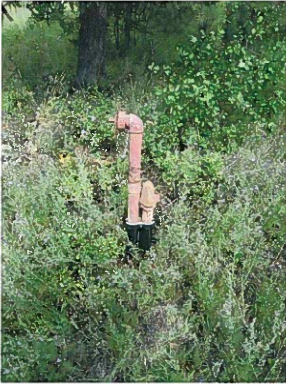
BWS Unused Fire hydrant
