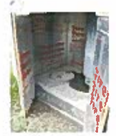
BWS Non- System Reservoir BLDG Interior.JPG
