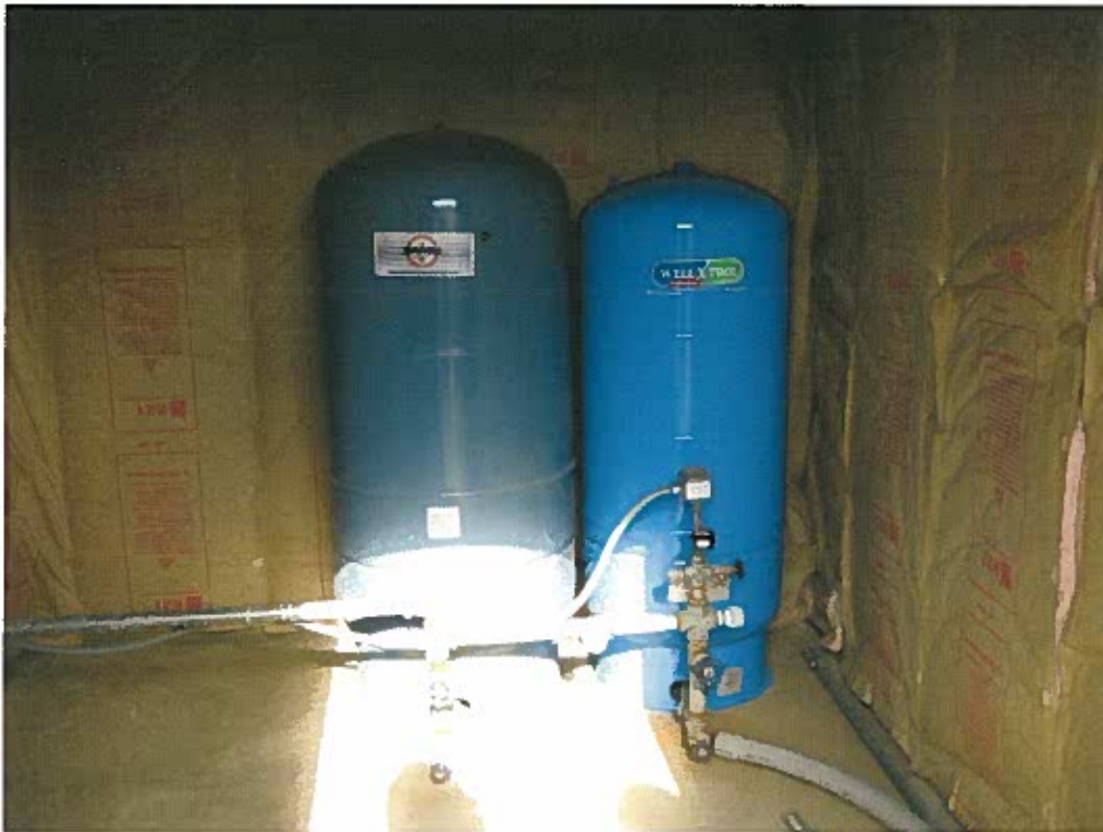
BWS Well House Pressure Tanks
