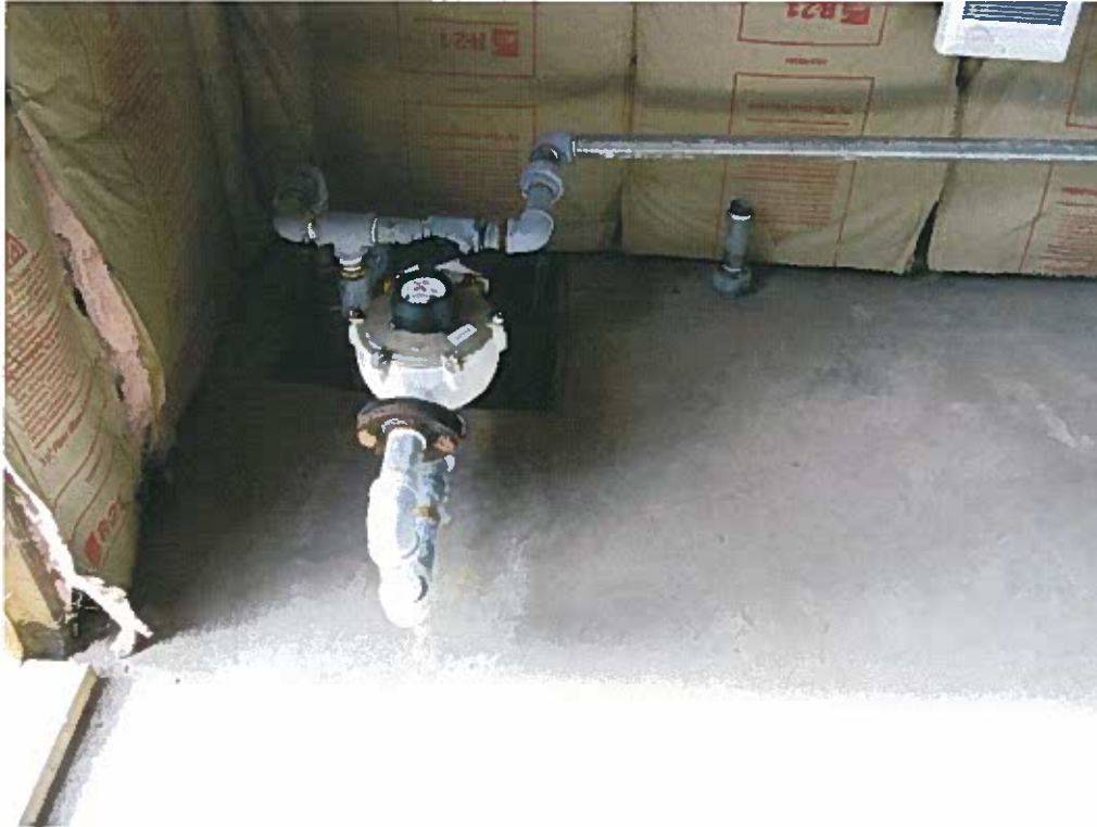
BWS Recordall Flowmeter Location
