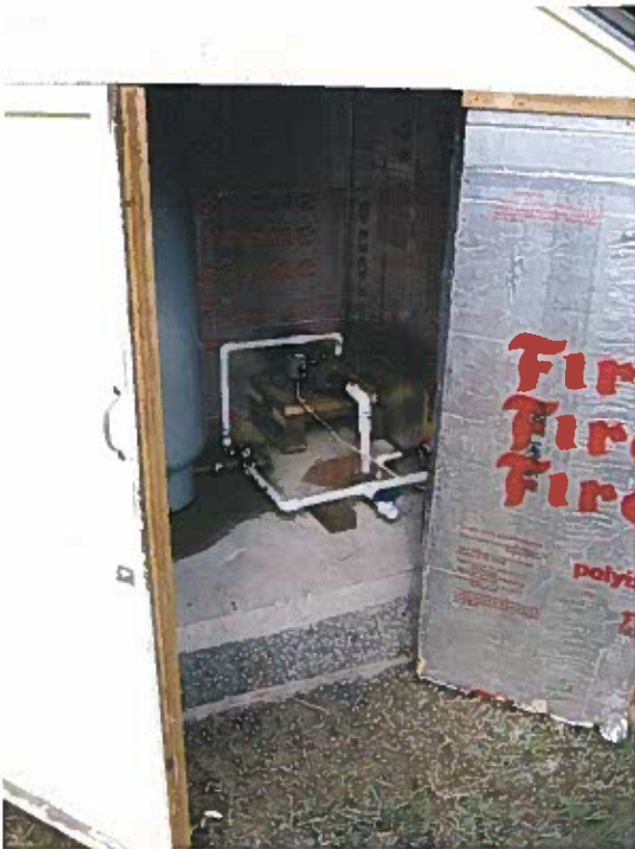
BWS- Non-System Reservoir BLDG Pump
