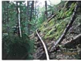
PIPE FROM LINDSEY CREEK TO POND 1
