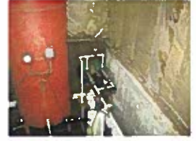
95-8999 Pumphouse Tank & Pumps.JPG
