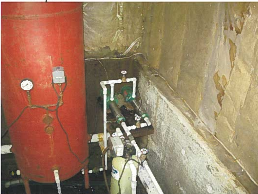
95-8999 Pumphouse Tank & Pumps
