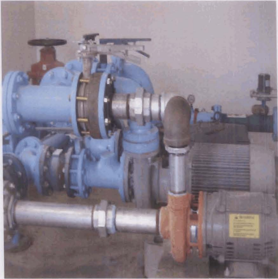
Well #1 E0006705 10 hp 3 Booster Pumps (10hp, 15hp, 25hp)
