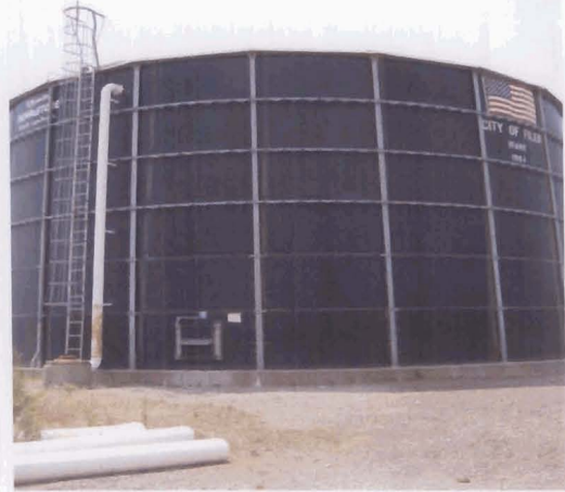
600,000 gal storage tank Associated with well #1
