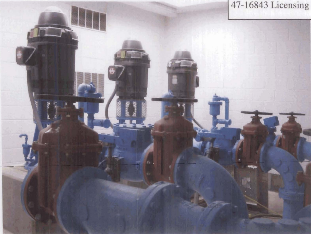
Boosters (50hp, 60hp, 100hp) located in new pump house from main storage tank (both shown in photo below). All 5 of the City of Filer's wells feed into the main storage tank and then are pumped via the boosters to the service area.
