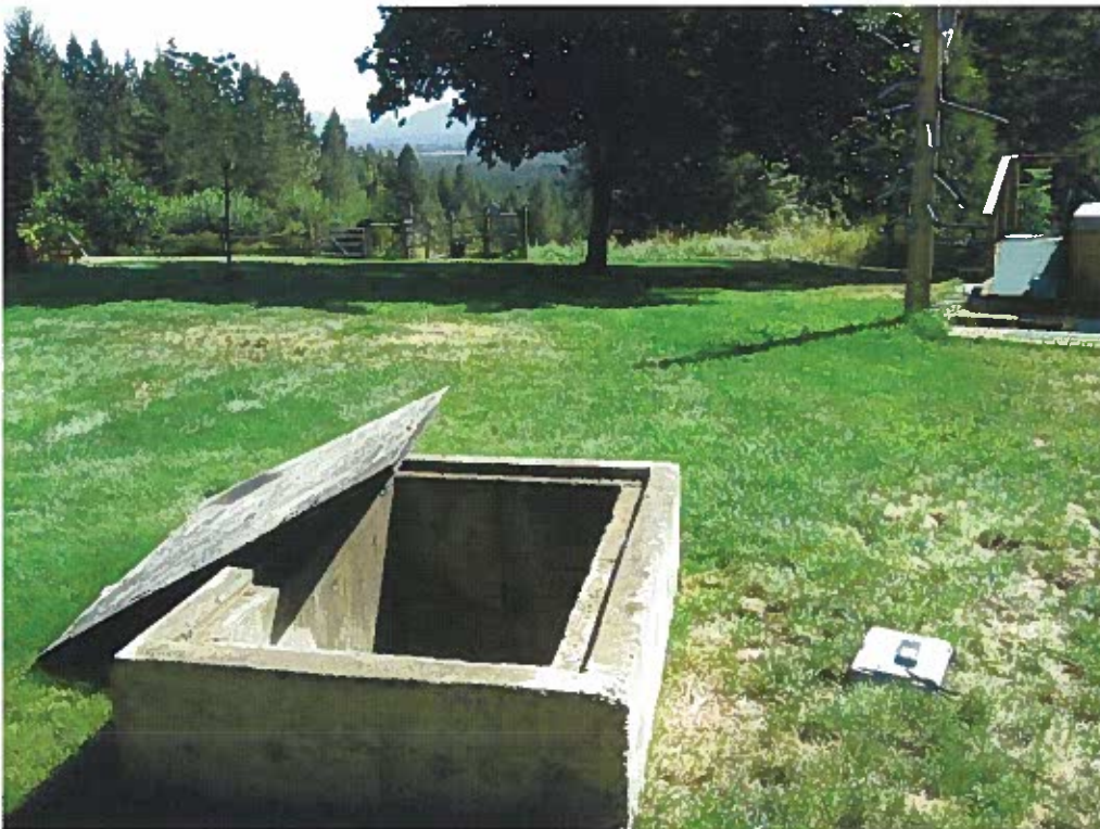
95-8998 Valve Box near Well & B & B
