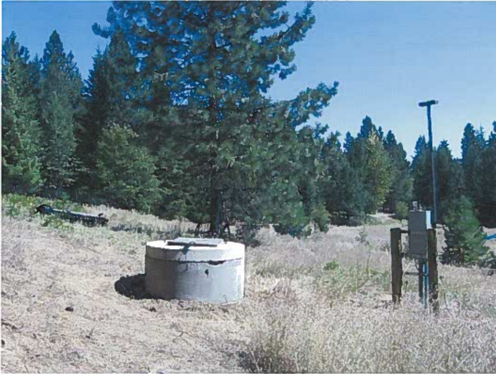
95-8998 East Concrete Vault View North
