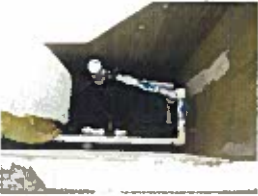
95-8998 Valve Box Interior.JPG
