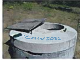
95-8998 East Concrete Vault & Spigot near Cabin Drive....
