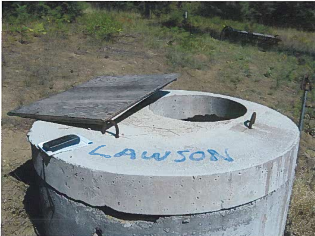
95-8998 East Concrete Vault & Spigot near Cabin Drive
