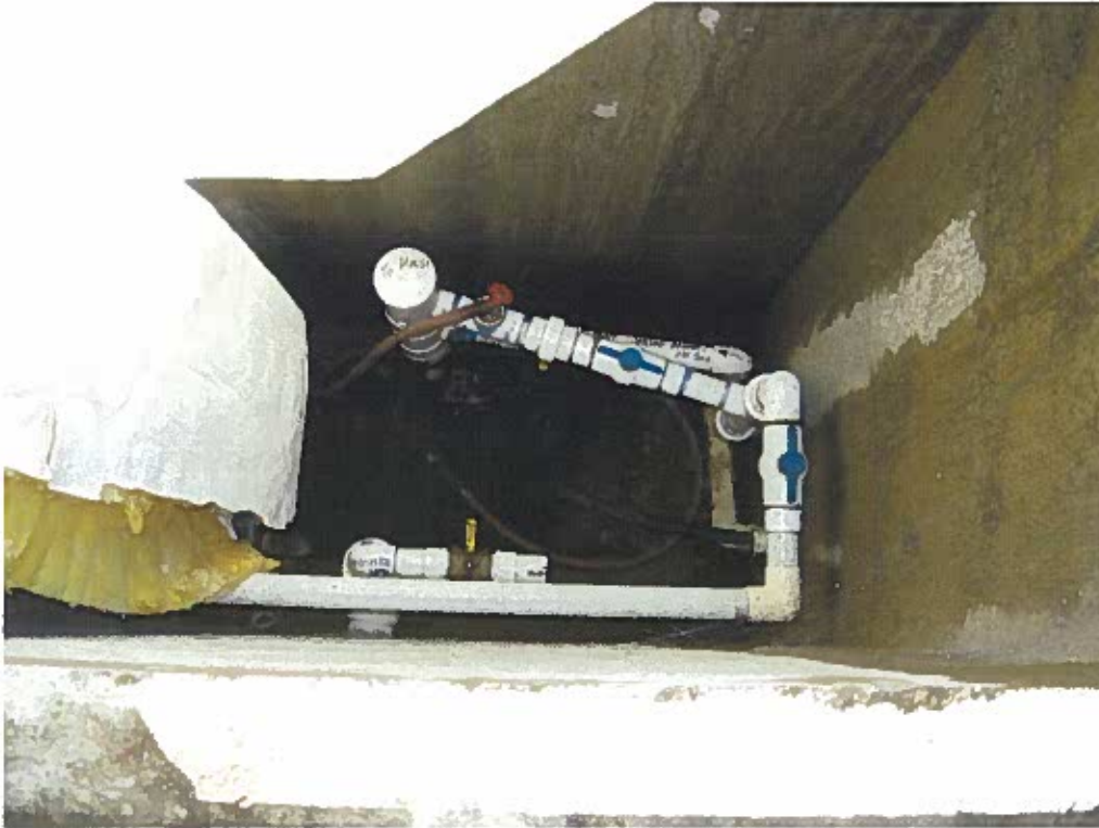
95-8998 Valve Box Interior
