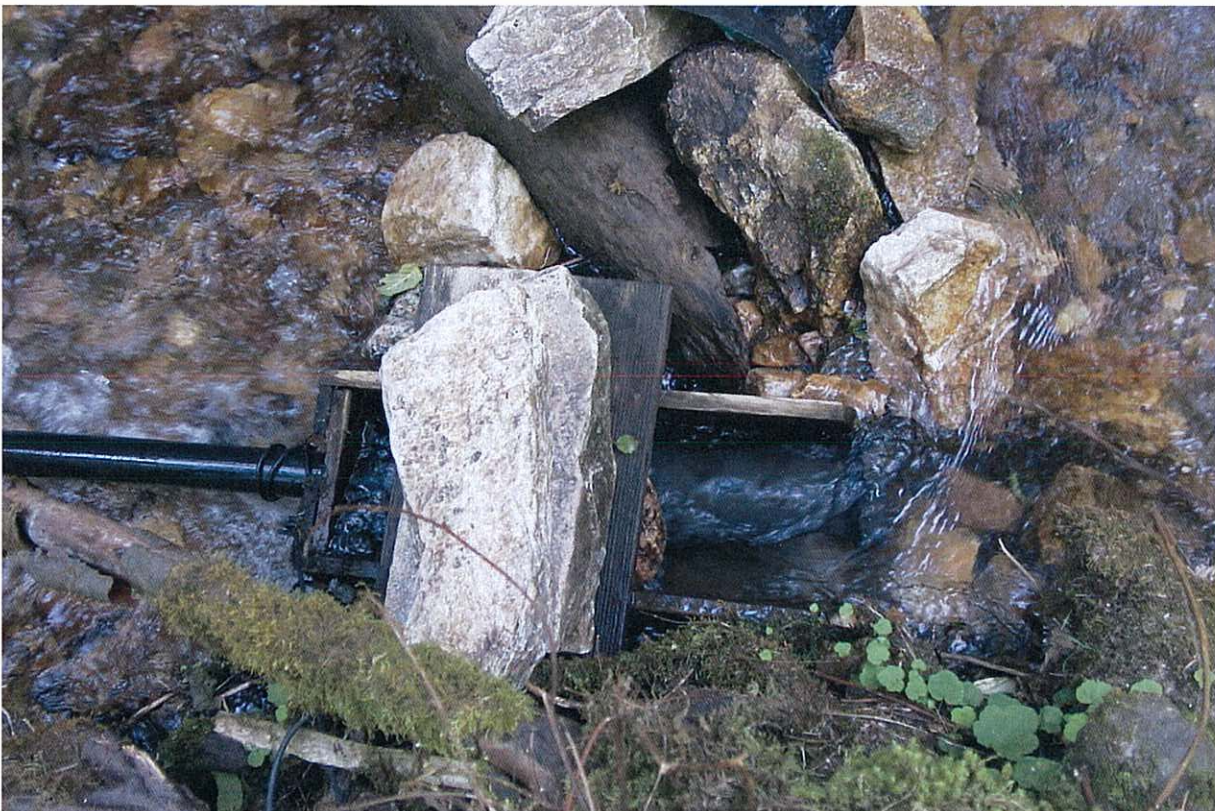
FIGURE 2: Diversion box, 4" mesh-screened intake, and 2" PVC pipeline.
