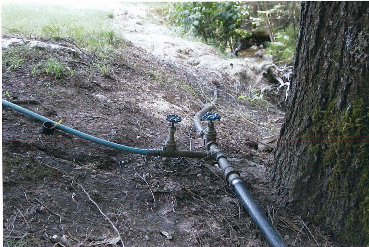
FIGURE 4: 2" pipeline, control valves, and reduction to hoses. View facing downhill, Little Smith Creek on right.
