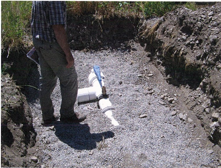
Figure 3. Valve installed in community line to accommodate licensing examination. Outlet pipe is next to Tim's feet. Directly upstream of valve and outlet is a location for a measuring device.
