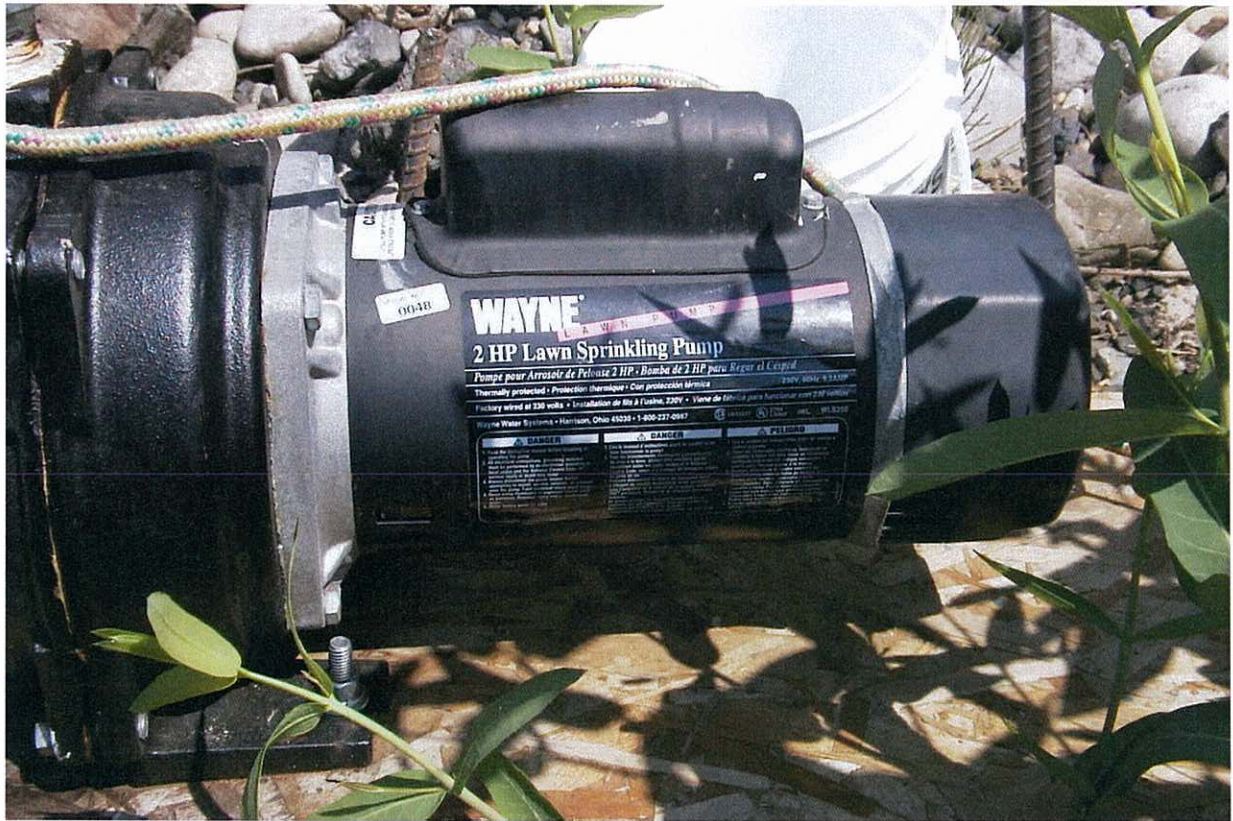
FIGURE 3: Close-up of pump.
