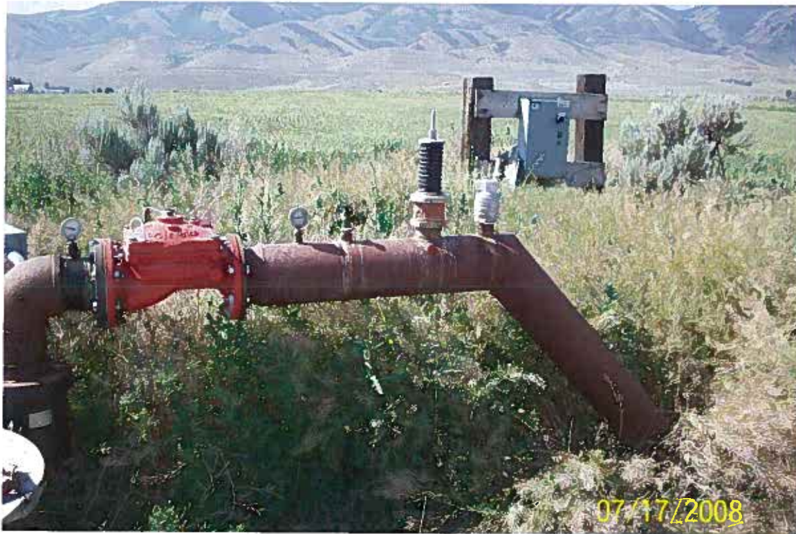
Photo #1 - Pump system N 42° 07.182' W 112° 20.501'
