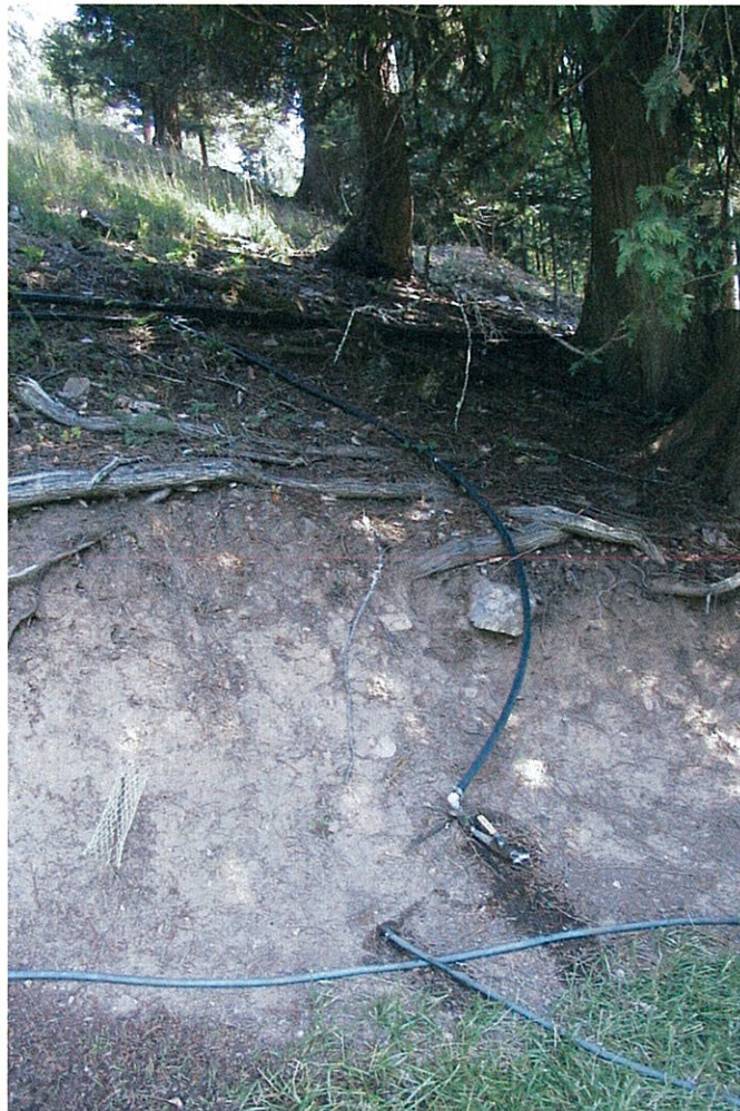
FIGURE 2: 2" pipeline traversing hill slope with delivery line, control valve, and garden hose to sprinkler.
