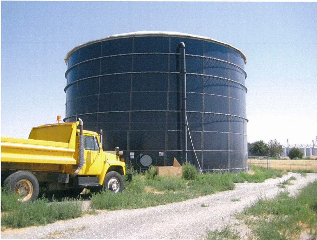
600,000 gallon storage tank that the five pumps feed into.
