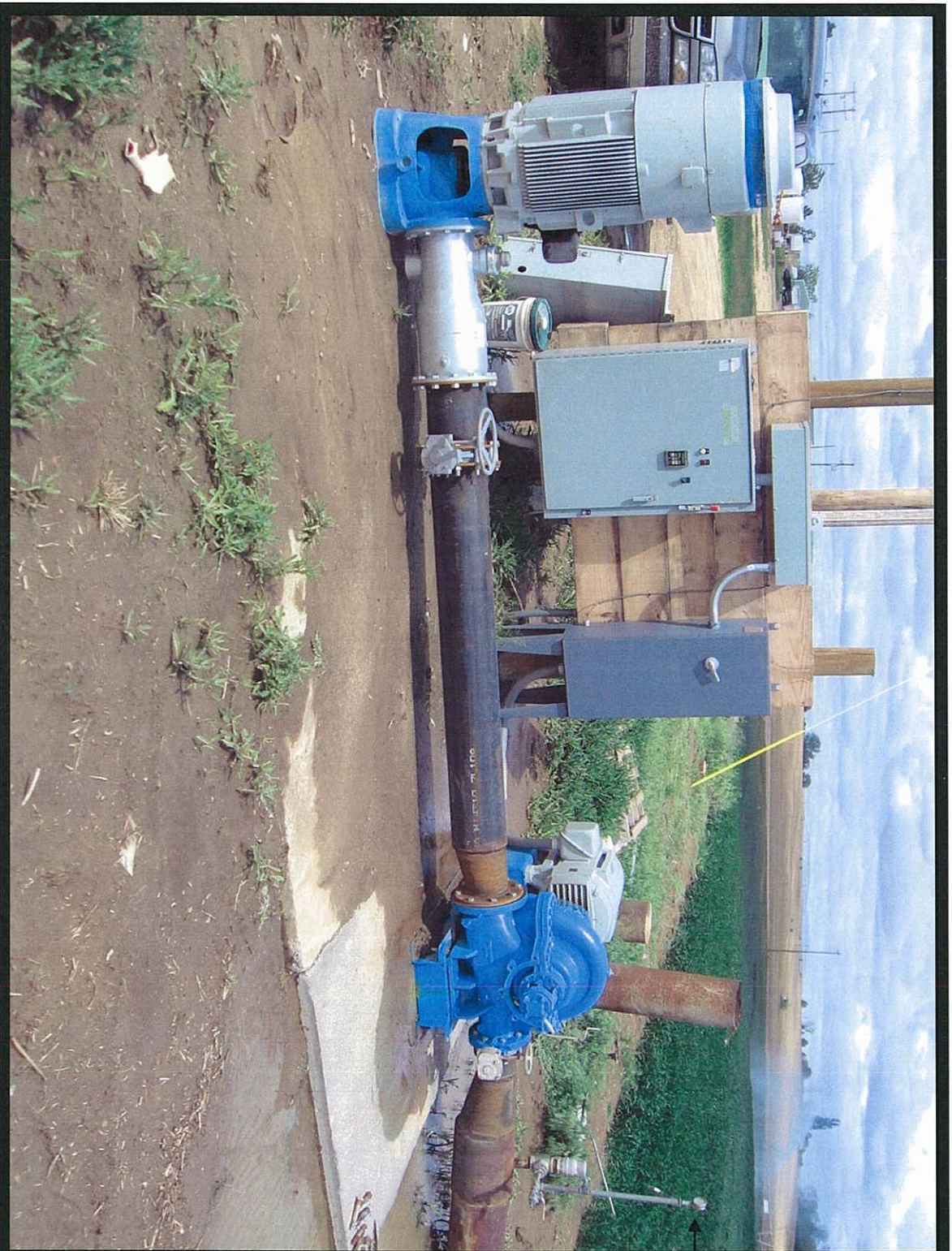
16" East Well, 150 HP Pump, 125 HP Booster
