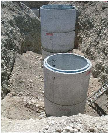
Lift Station in foreground, surge tank in background.
