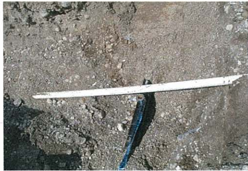
6" water main below pressure sewer. Told A+ to sleeve the sewer line.
