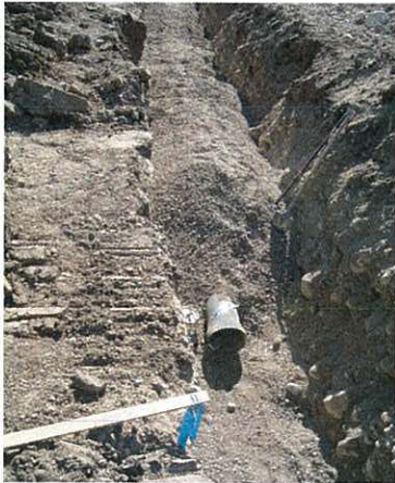
Satisfactory bedding, and tracer wire
