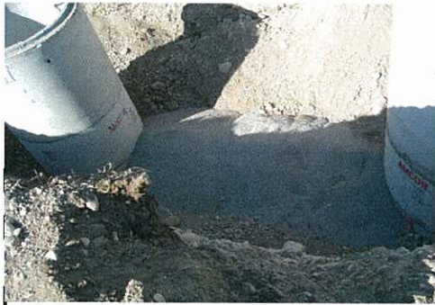
Back fill of Lift station Compaction needed
