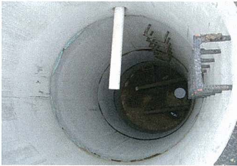
Picture looking down into lift station
