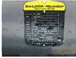
PUMP MOTOR INFORMATION.JPG
