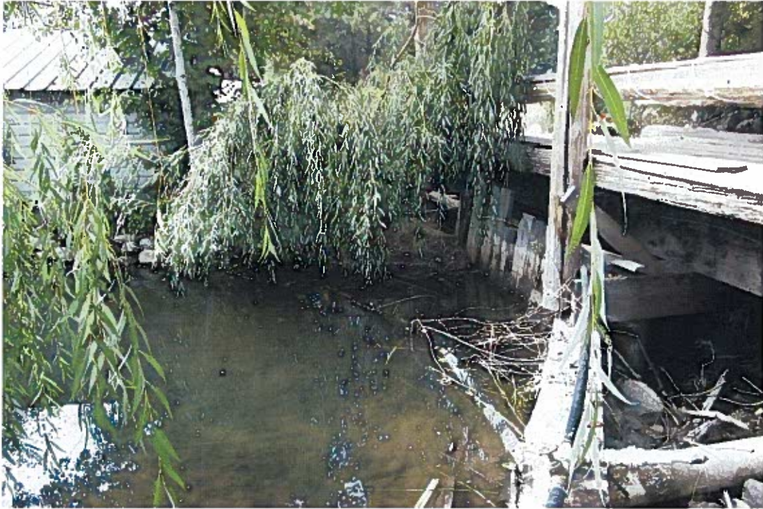
95-8858 Pump House Rathdrum CR Dam
