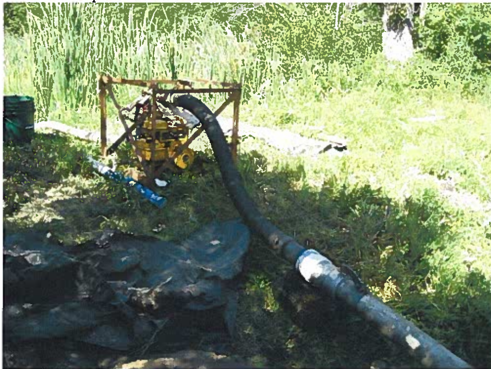
95-8457 AUG 08 Pump Pond 3
