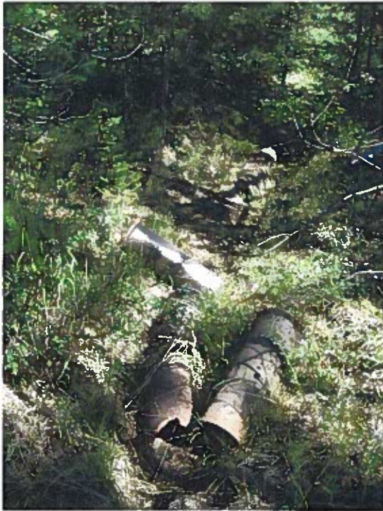
95-8457 Broken Pipe Ditch Stream 2
