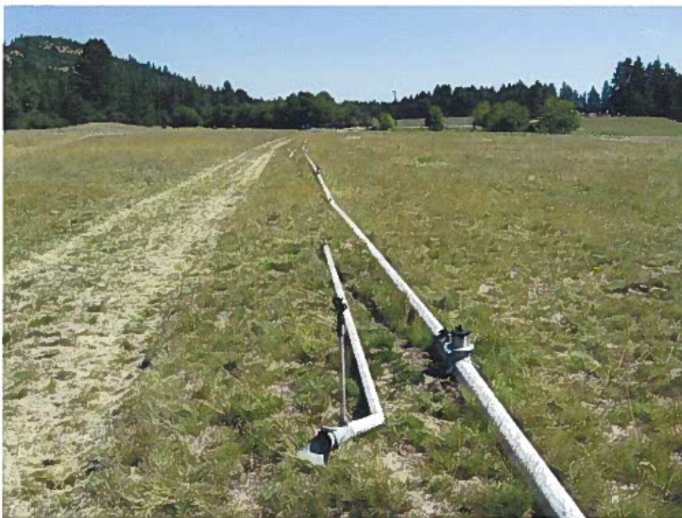
95-8457 Pipeline North to POU
