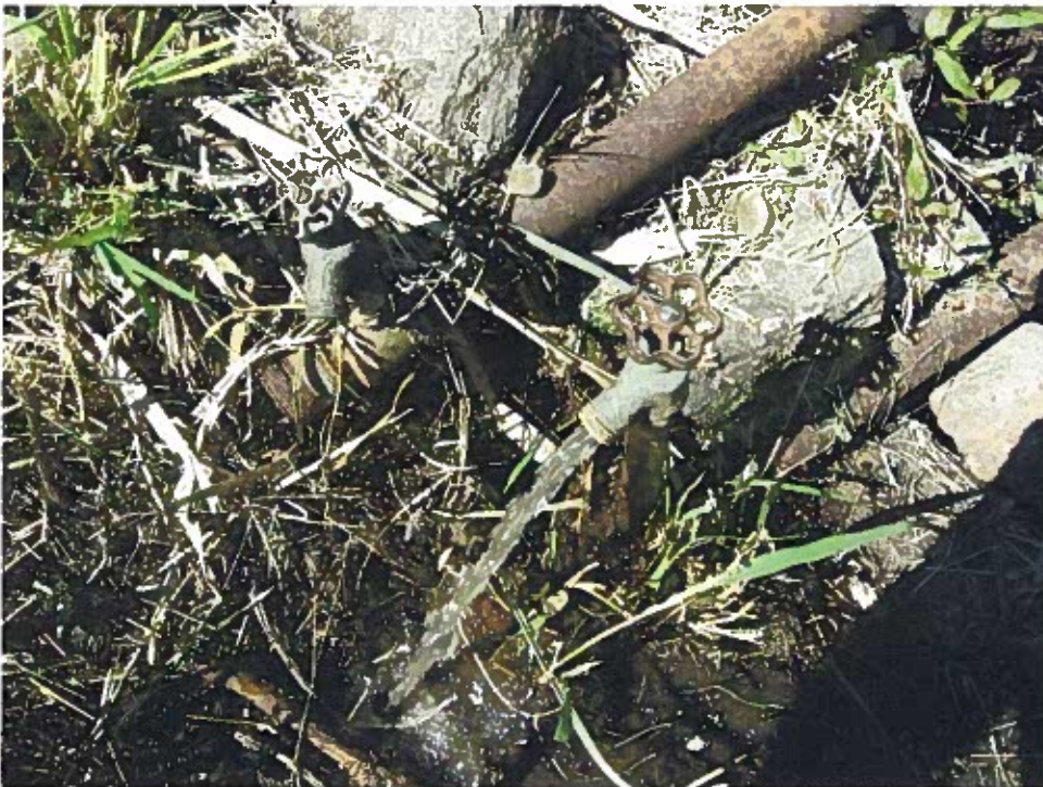
95-8457 Faucets Below Pond 3
