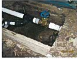
VALVE FOR POWER.JPG
