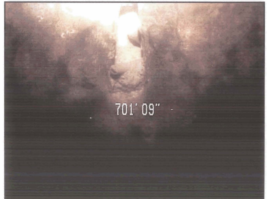
Side view still photograph of the inside wall of the ISCI Well #3 steel casing showing corrosion and formation sand visible through a hole in the casing at ~701 feet below land surface.
