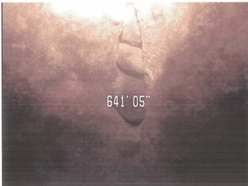
Side view still photograph of the inside wall of the ISCI Well #3 steel casing showing a sand-widened perforation with gravel particles visible through the hole in the casing at ~641 feet below land surface.
