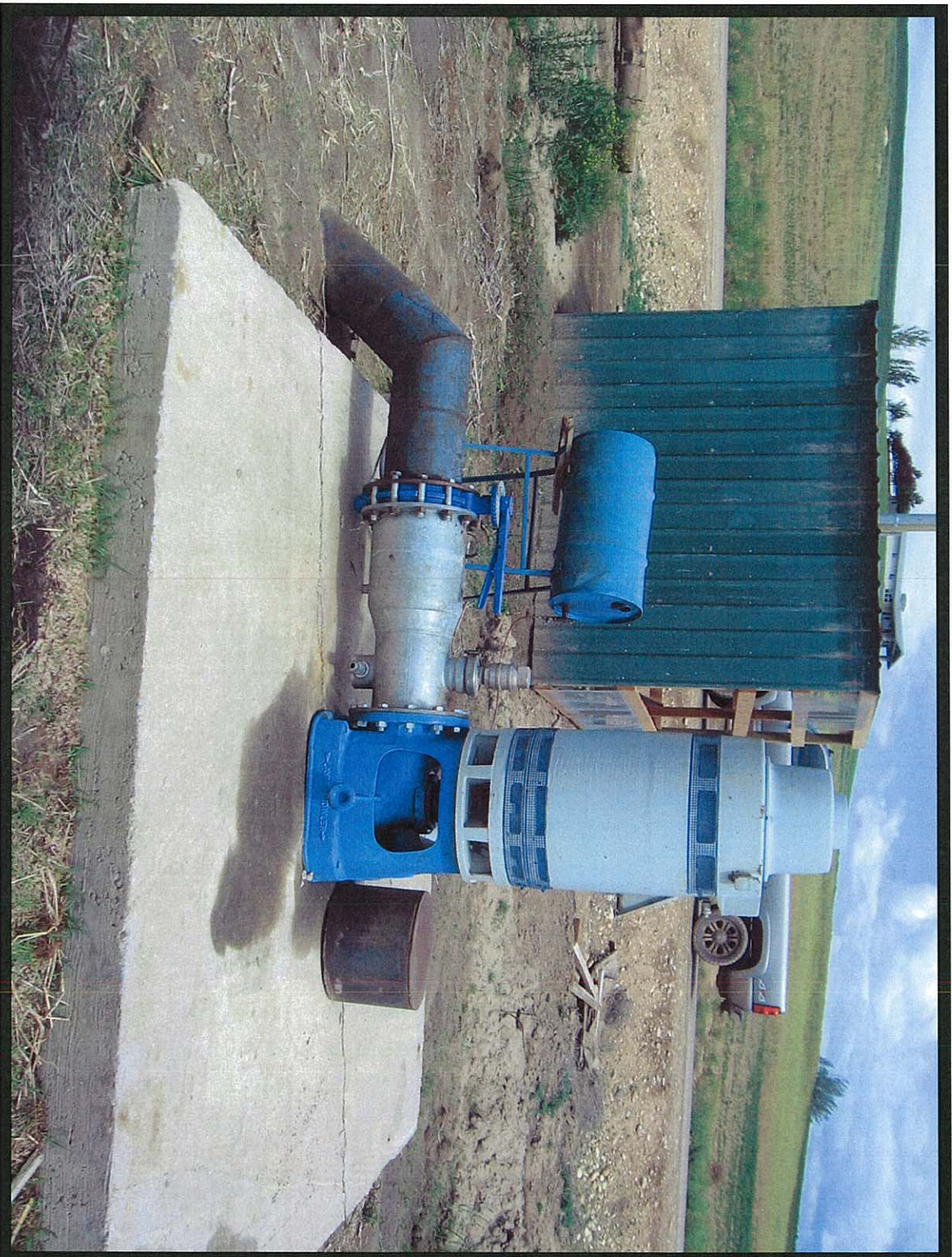
16" West Well, 200 HP Pump
