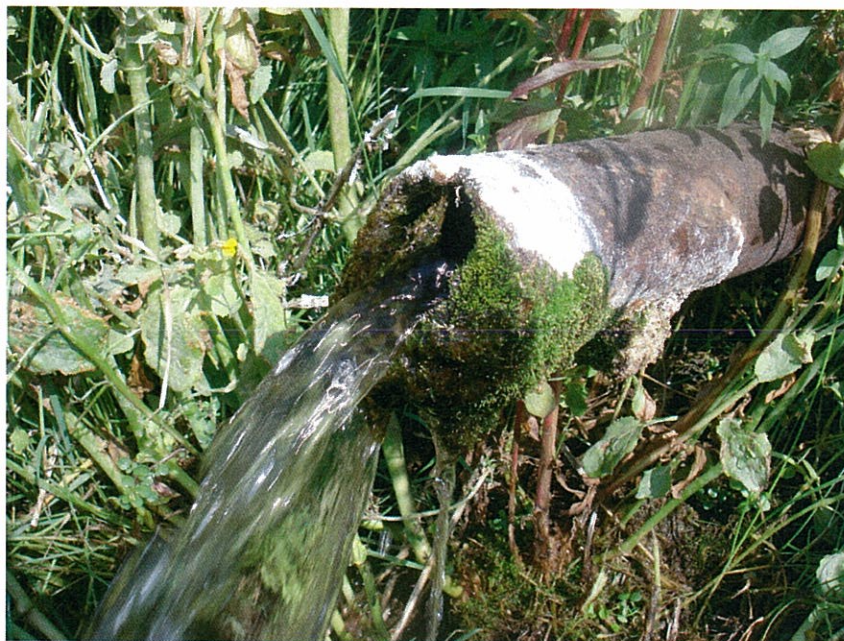
- 2.5 inch steel pipe that intercepts spring
