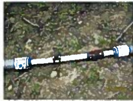
FLOW METER AND SHUT OFF VALVE.JPG
