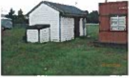
PUMP HOUSE WELL #1.JPG
