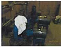
BOOSTER PUMPS FROM STORAGE.JPG
