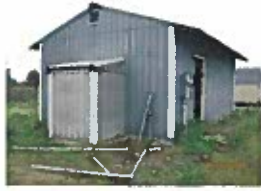
PUMP HOUSE WELL #2.JPG
