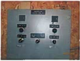
BOOSTER PUMP CONTROL PANEL.JPG
