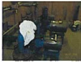
BOOSTER PUMPS FROM STORAGE.JPG
