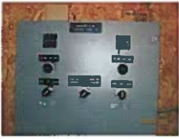
BOOSTER PUMP CONTROL PANEL.JPG
