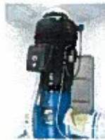
PF Well 8 Pump and Motor.JPG
