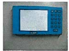
PF Well 7 Telemetry.JPG
