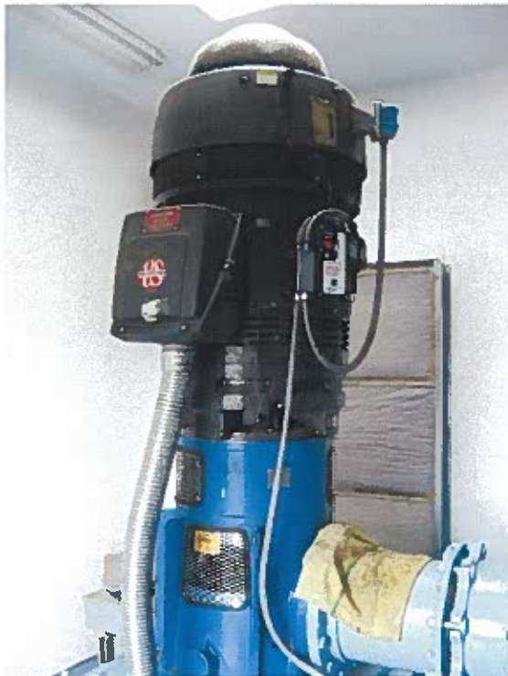
PF Well 8 Pump & Motor
