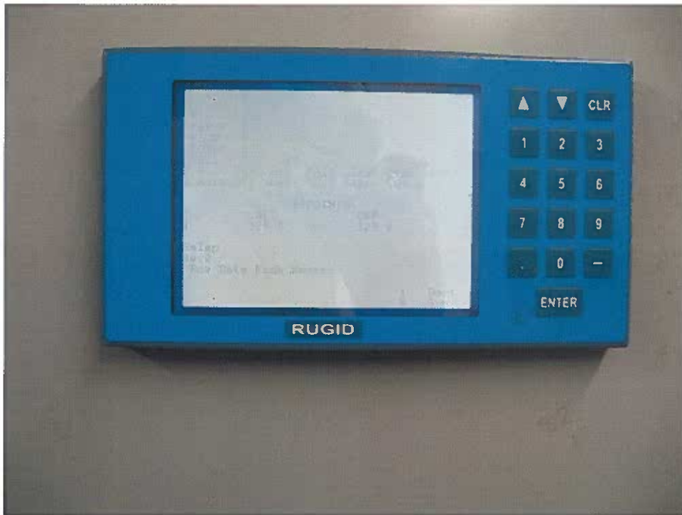
PF Well 7 Telemetry
