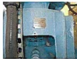
PF Well 9 Pump Data.JPG
