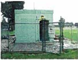
PF Well 1 & Irrigation Pump.JPG
