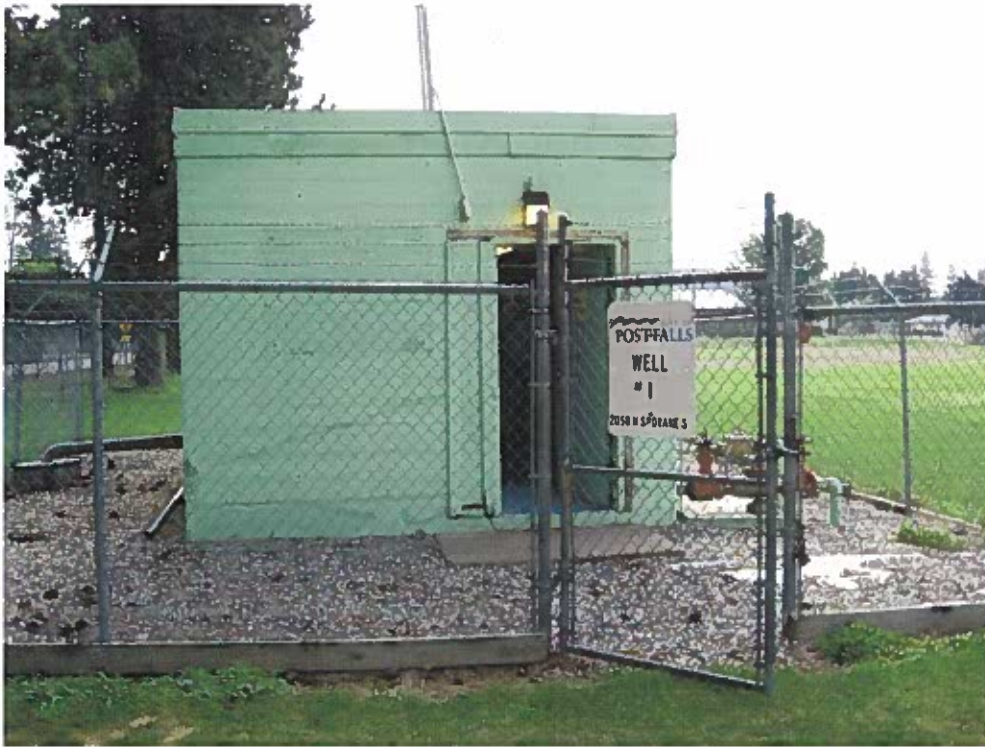
Well 1 and Irrigation Pump
