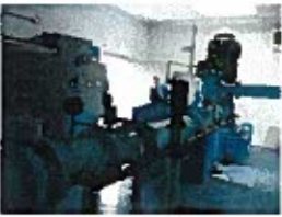
PF Well 8 Inside.JPG
