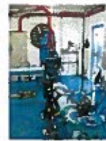
PF Well 7 Inside.JPG
