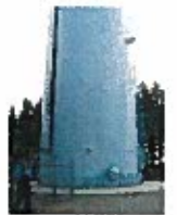
PF Wells 5 & 7 Reservoir.JPG
