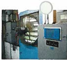
PF Well 1 Telemetry.JPG
