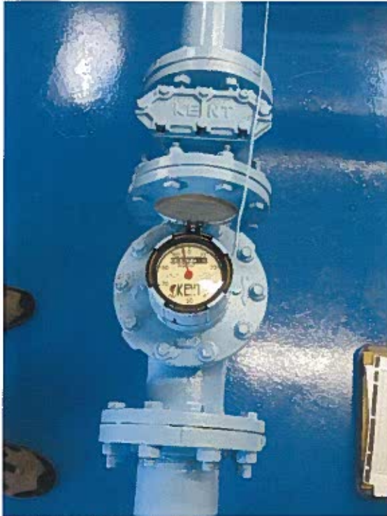
95-8768 Well House Flowmeter
