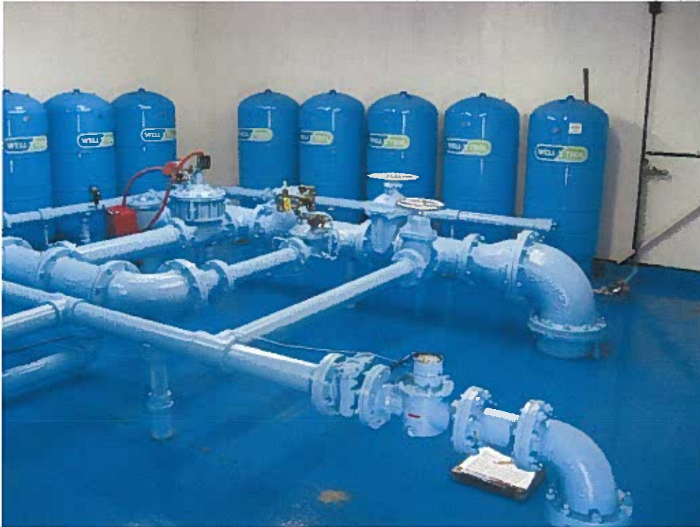
95-8768 Wellhouse Inside & Flowmeter
