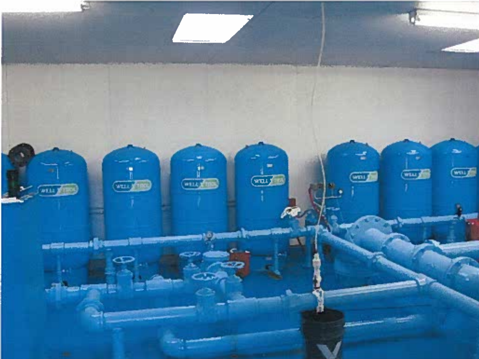
95-8768 POD Pressure tanks
