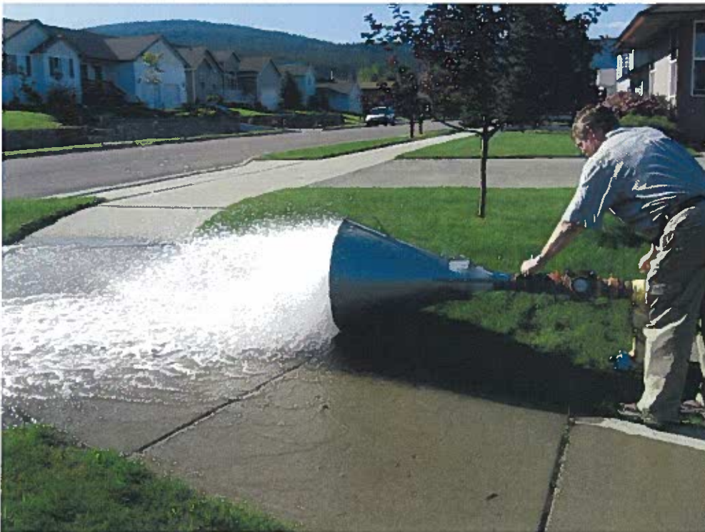
95-8768 Fire Well Test & POU
