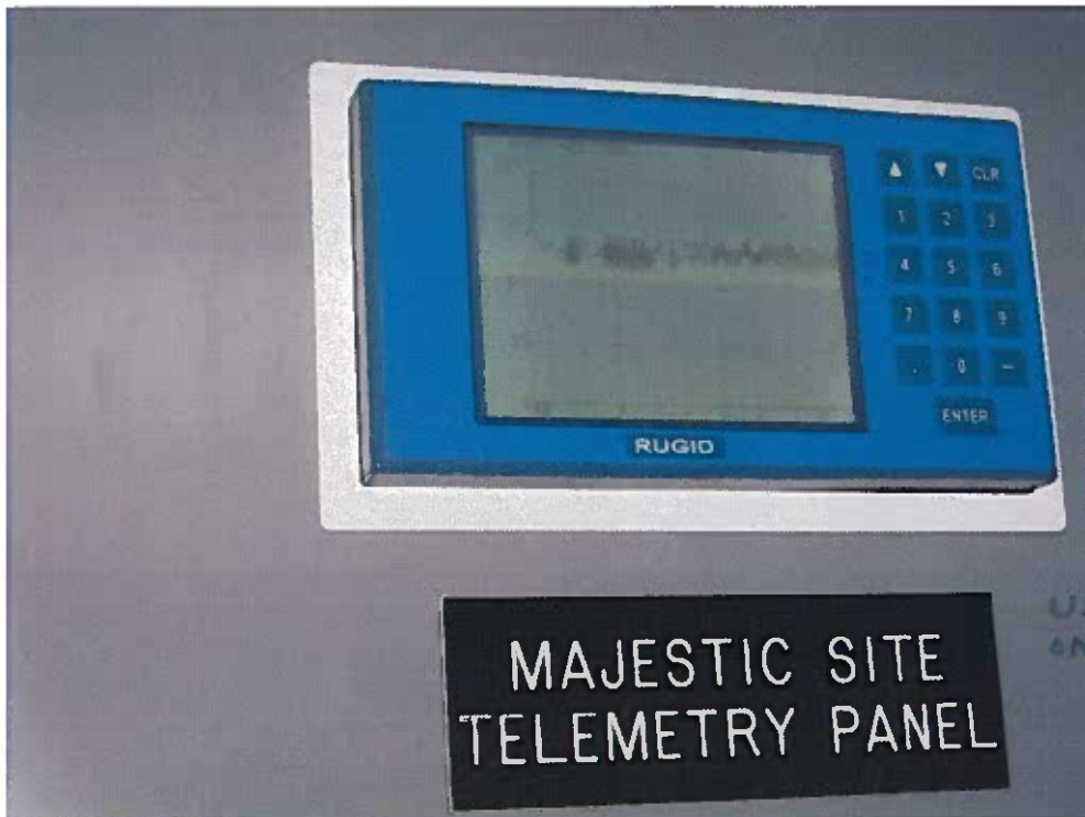
95-8768 POD Telemetry Panel
