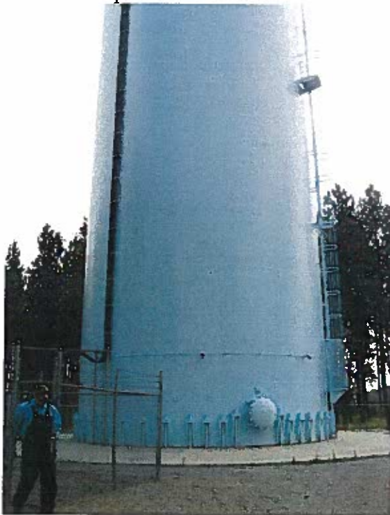
PF Wells 5 & 7 Reservoir
