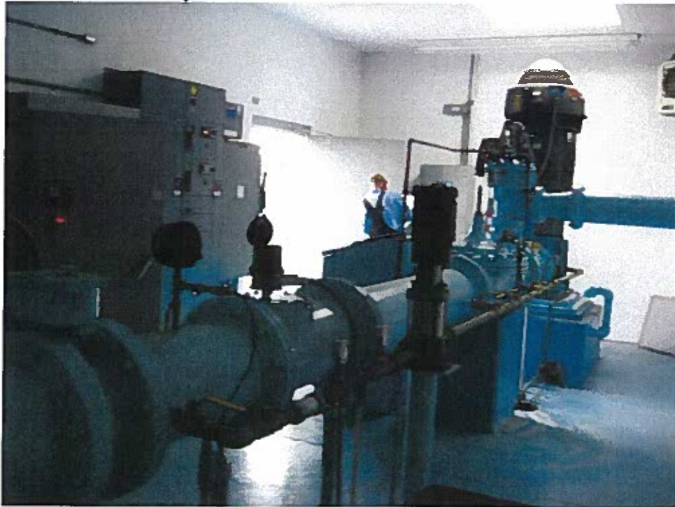
PF Well 8 Inside
