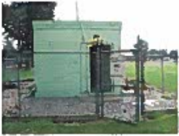
PF Well 1 & Irrigation Pump.JPG
