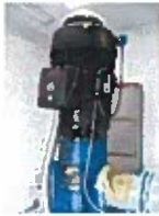
PF Well 8 Pump and Motor.JPG
