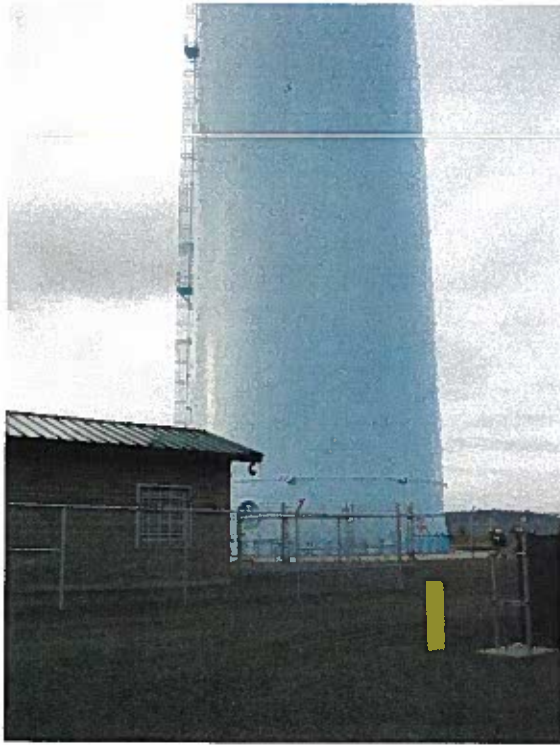
Well 9 and Reservoir
