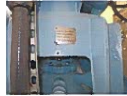
PF Well 9 Pump Data.JPG
