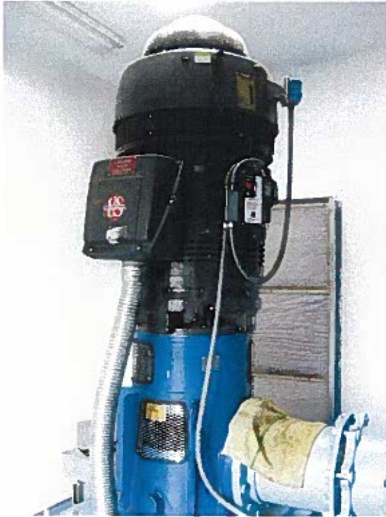
PF Well 8 Pump & Motor
