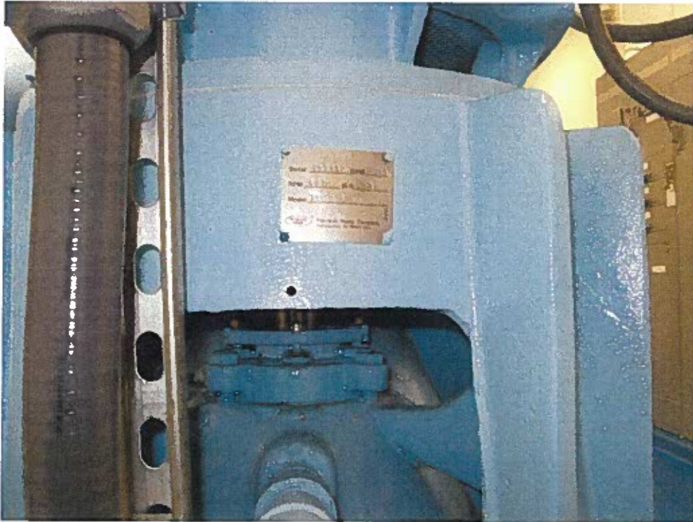
Well 9 Pump Data
