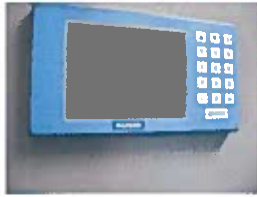
PF Well 8 Telemetry 1956 GPM.JPG
