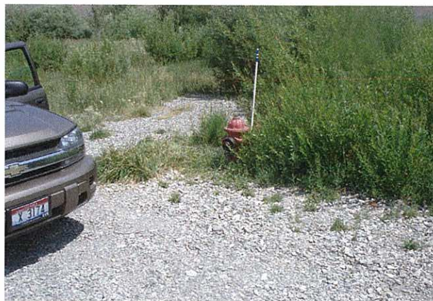
- Fire hydrant. Located next to road that wraps around west side of pond. Hydrant approximately 100 feet from pond.
