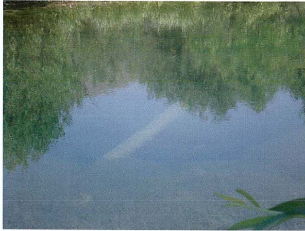
-Intake pipe for fire hydrant.
