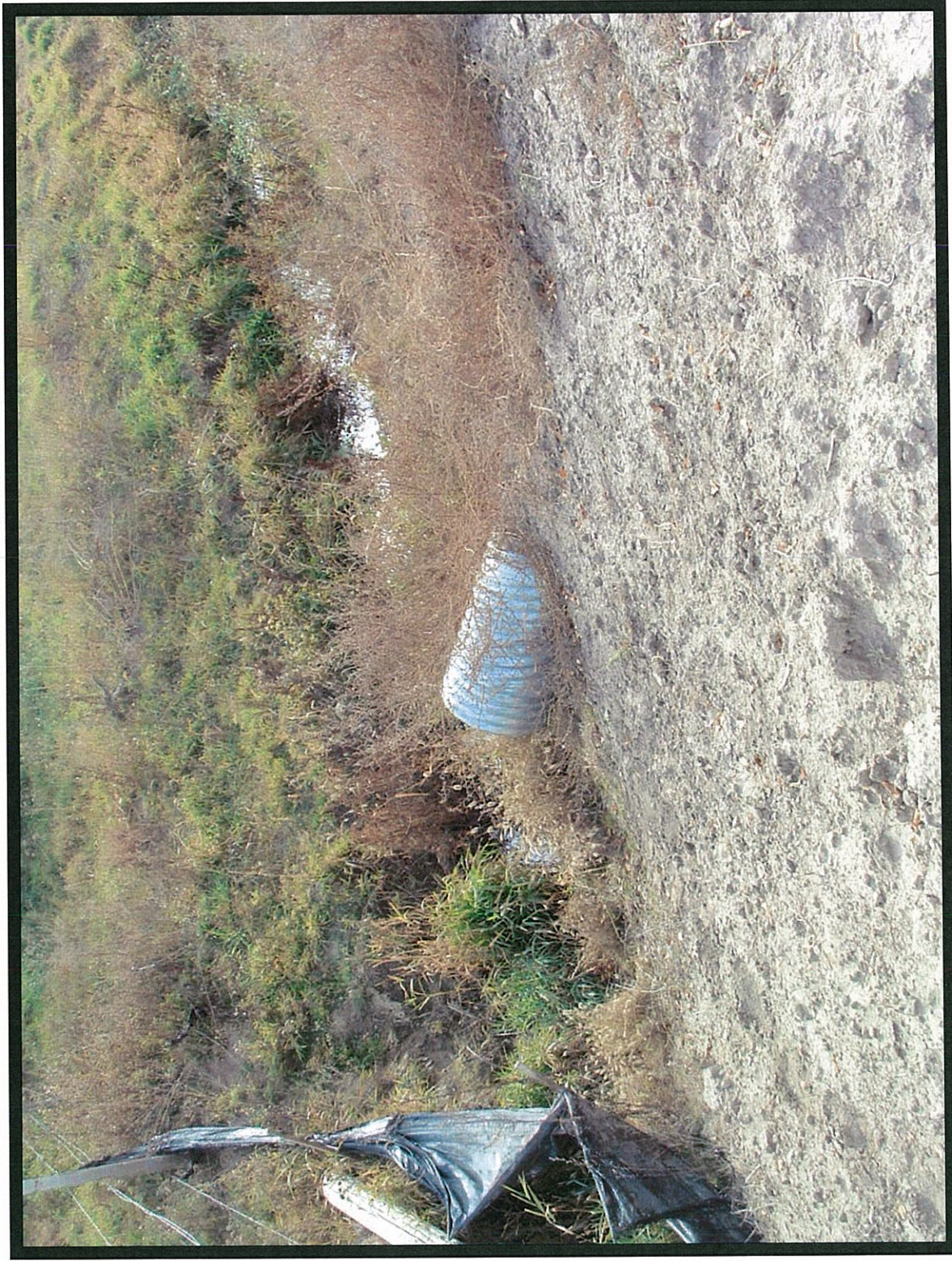
Overflow pipe to drain near Snake River
